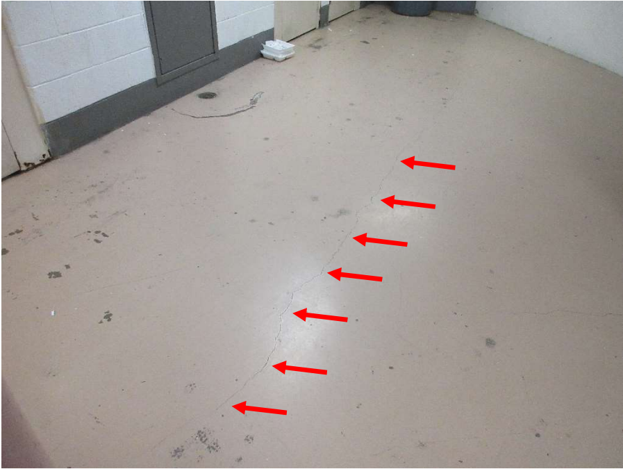
Photo 7 - Cracking in slab top surface at Level 13
