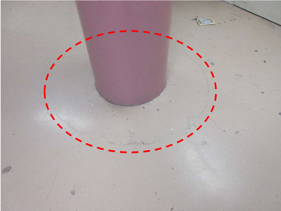
Photo 17 – Circular construction joint around column at Level 13
