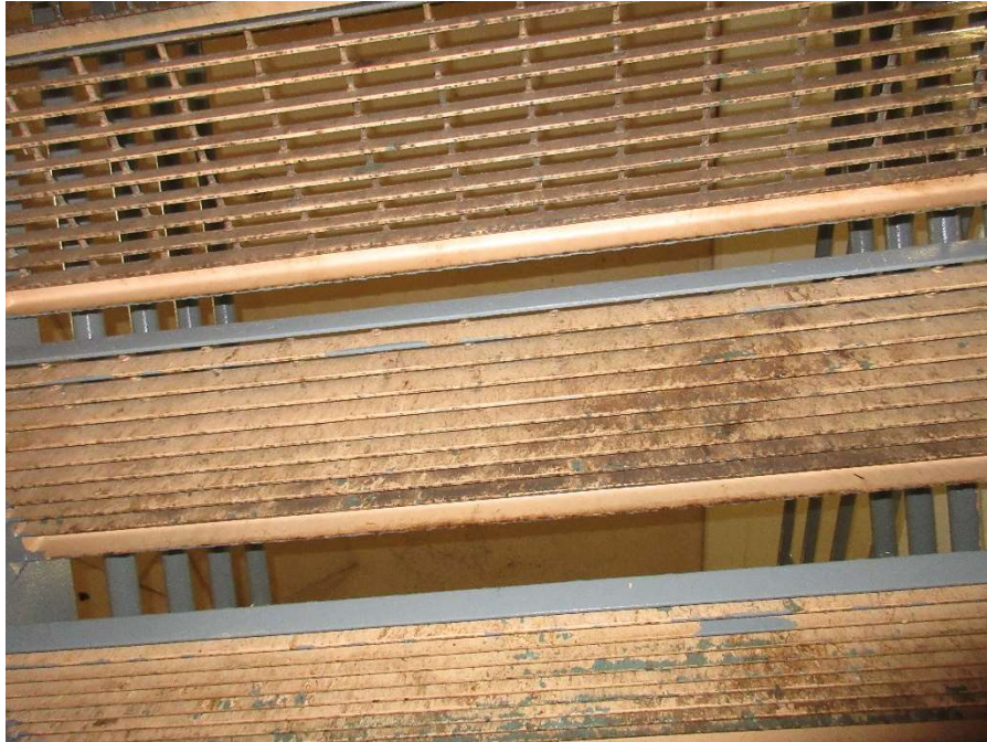
Photo 27 - Minor corrosion of steel treads at stair
