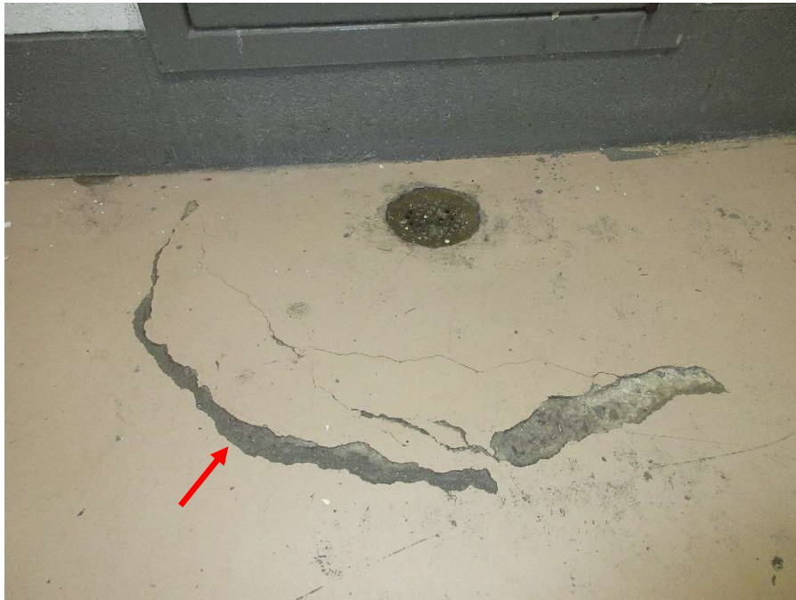
Photo 29 - Concrete damage near floor drain at Level 13
