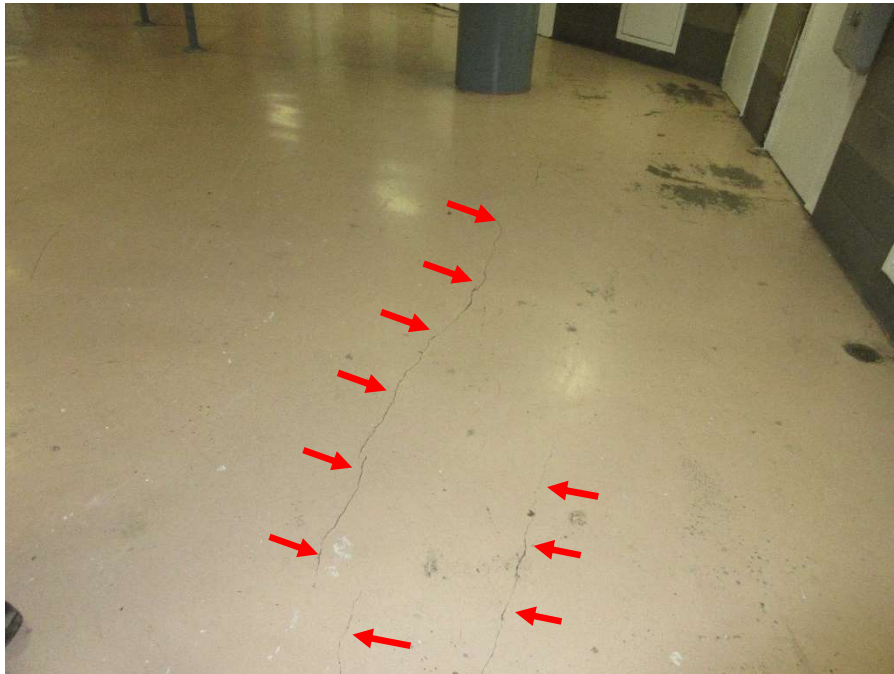
Photo 13 - Cracking in slab top surface at Level 8
