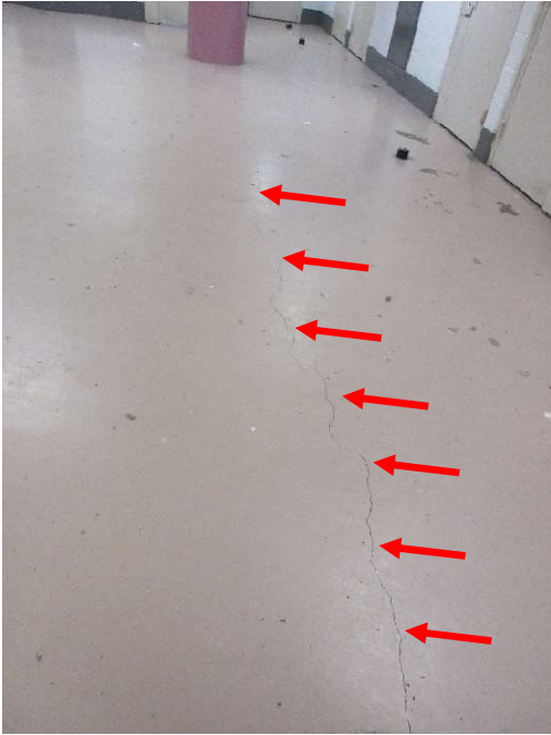
Photo 9 - Cracking in slab top surface at Level 13
