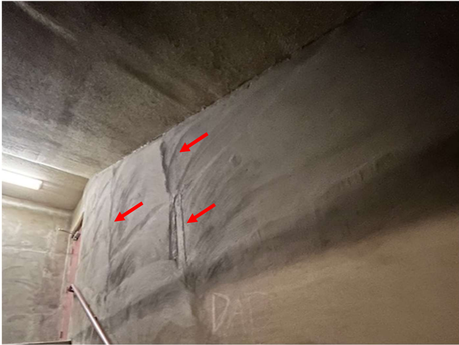
Photo 44 – Surface imperfections in stairwell wall
