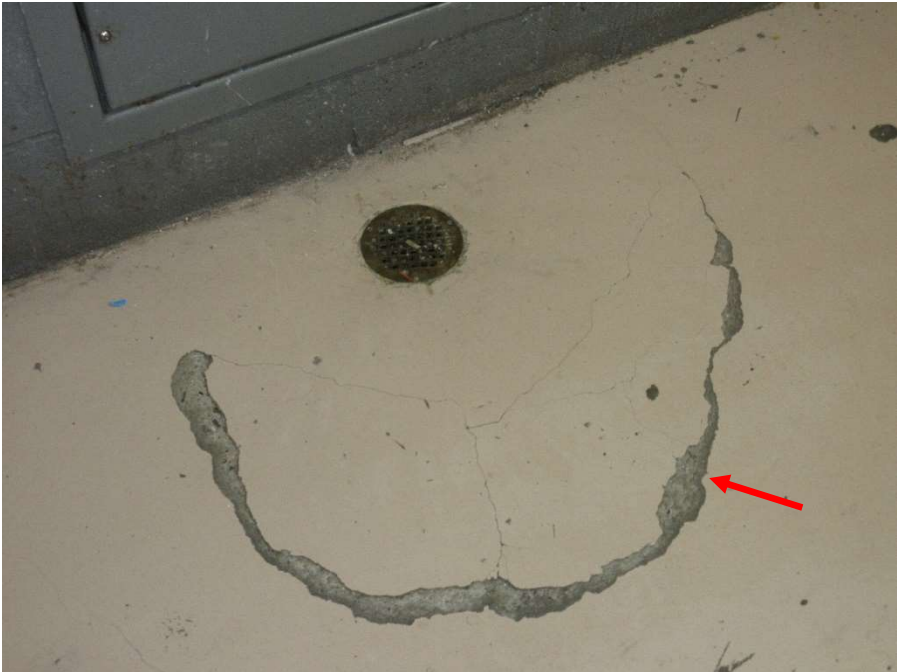
Photo 32 - Concrete damage near floor drain at Level 2
