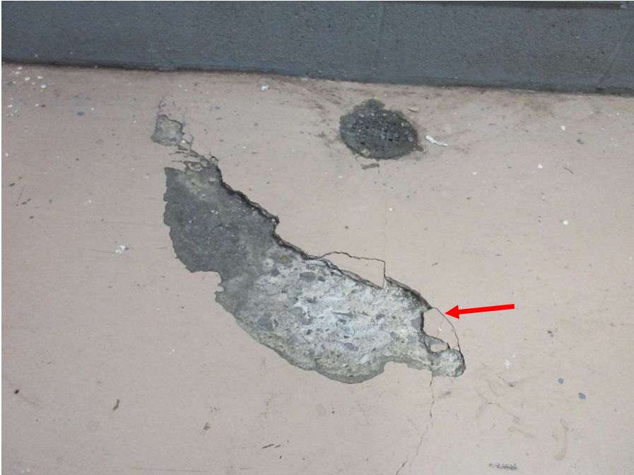
Photo 31 - Concrete damage near floor drain at Level 10
