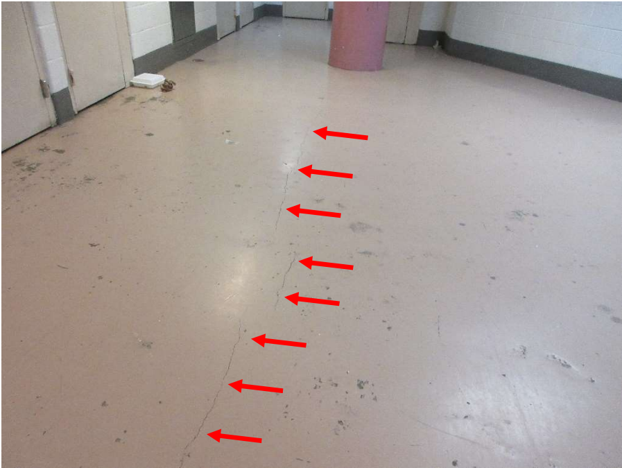
Photo 8 - Cracking in slab top surface at Level 13
