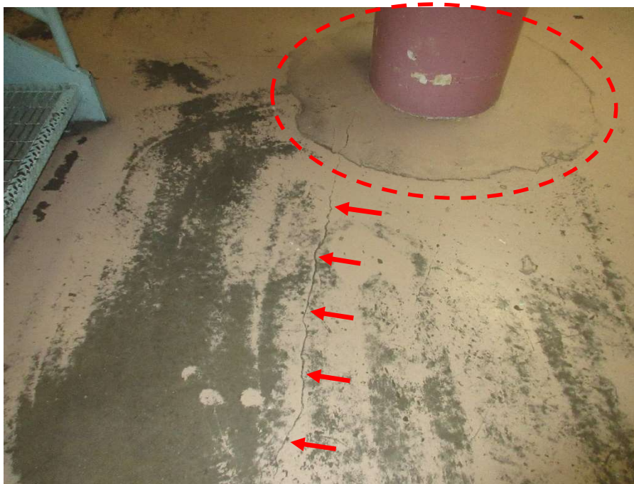
Photo 22 – Circular construction joint & cracks at Level 4
