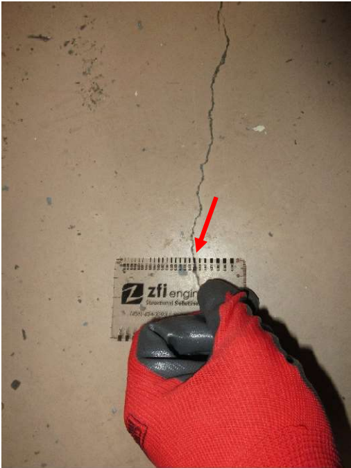
Photo 20 – Approximate width (0.040") of crack in slab top surface at Level 12
