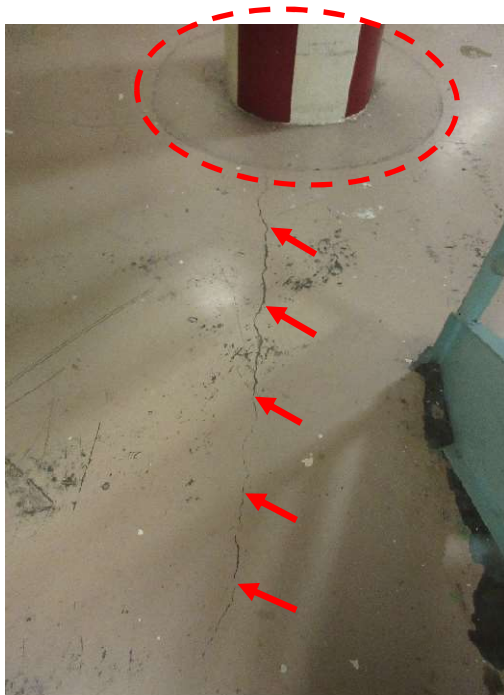
Photo 21 – Circular construction joint & cracks at Level 10
