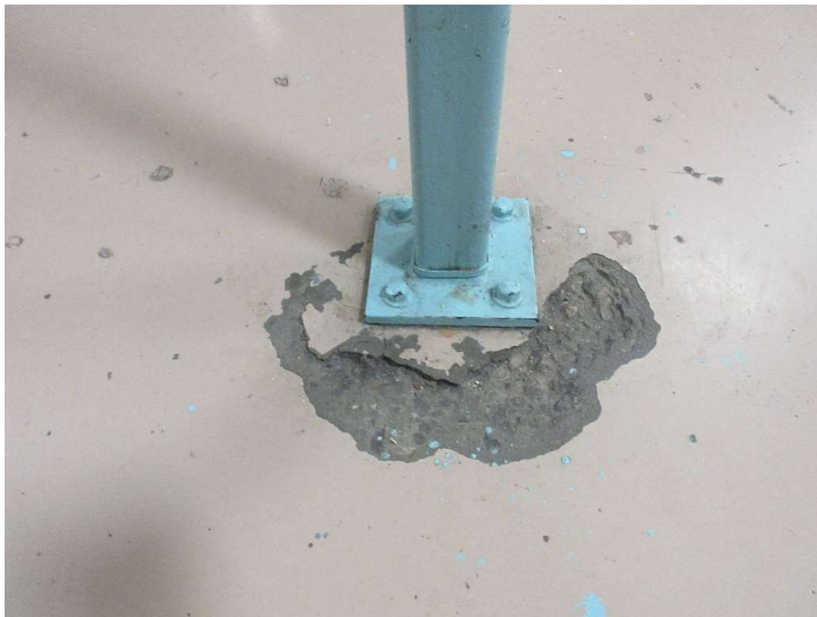
Photo 28 - Concrete damage at base of stair column
