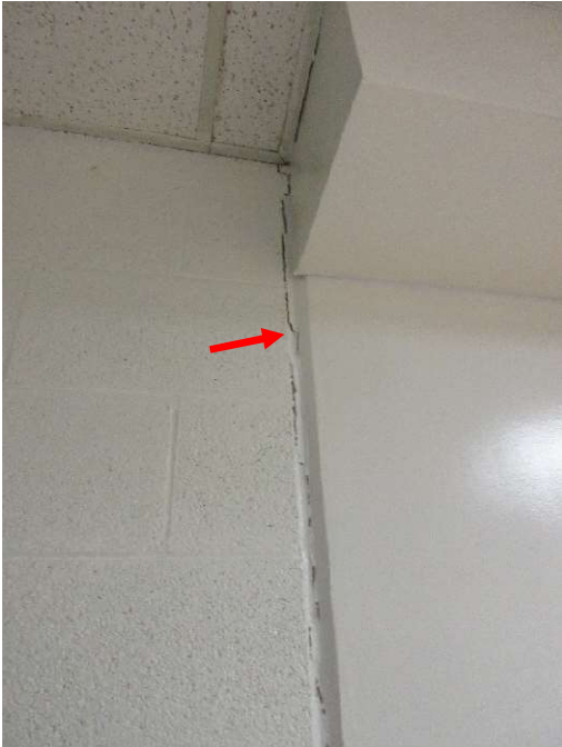
Photo 35 – Cracking in sealant of vertical joint at interior wall @ Level 13
