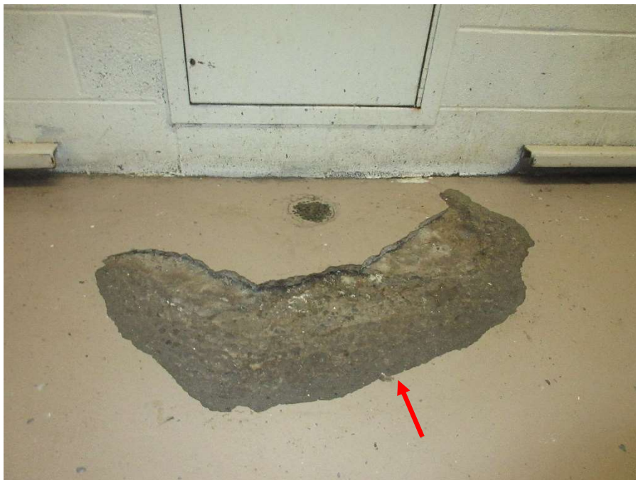
Photo 30 - Concrete damage near floor drain at Level 12
