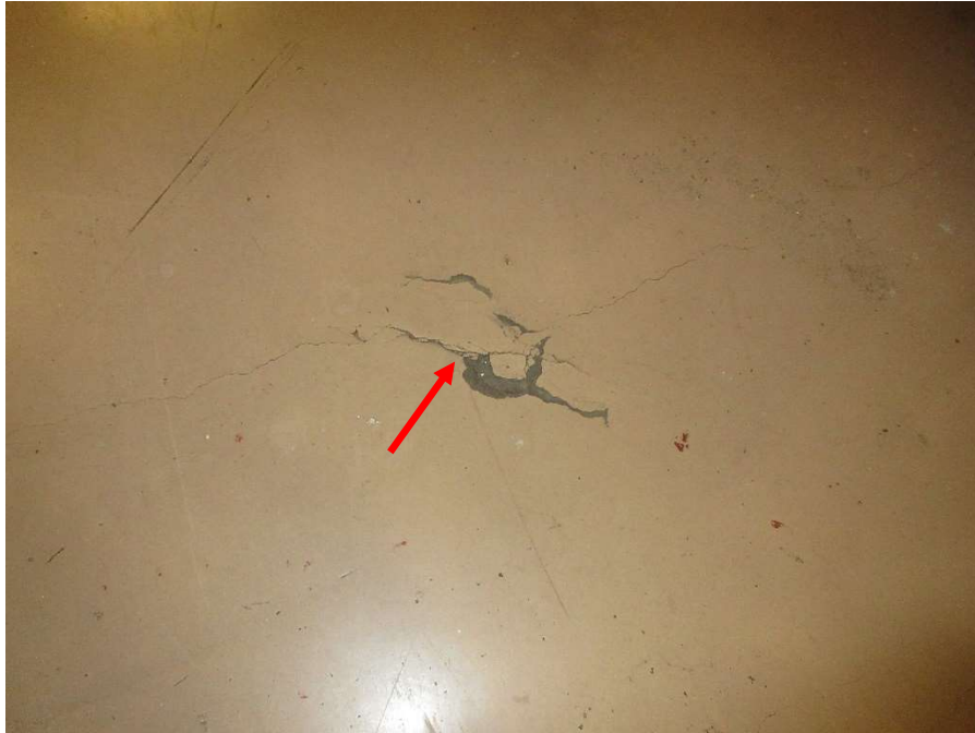
Photo 33 – Concrete delamination along crack at Level 10
