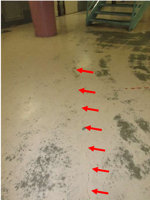
Photo 15 - Cracking in slab top surface at Level 4
