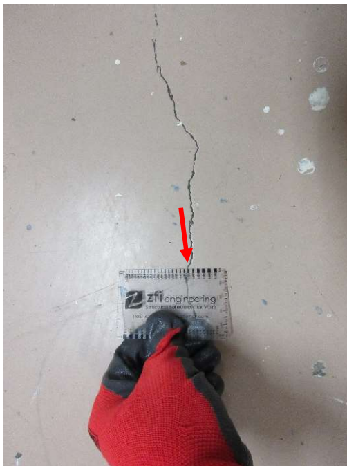
Photo 14 - Approximate width (0.050") of crack in slab top surface at Level 8
