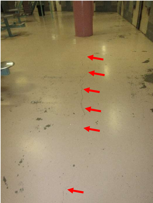
Photo 12 - Cracking in slab top surface at Level 10
