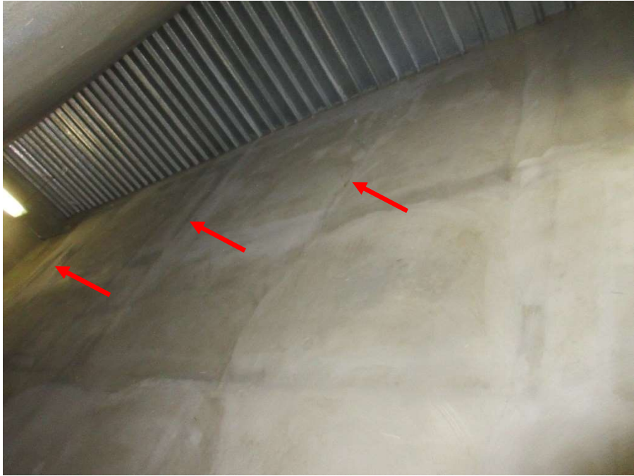
Photo 43 – Surface imperfections in stairwell wall
