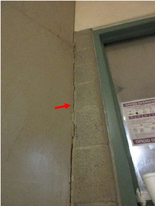
Photo 36 – Cracking in finishes at interior wall @ Level 4
