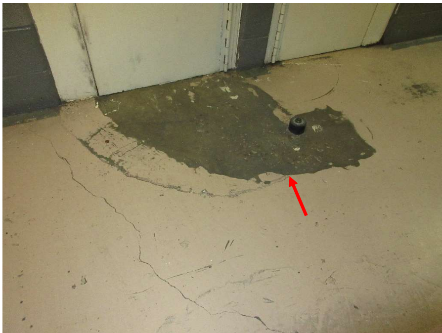
Photo 34 – Significant abrasion of concrete surface at Level 4
