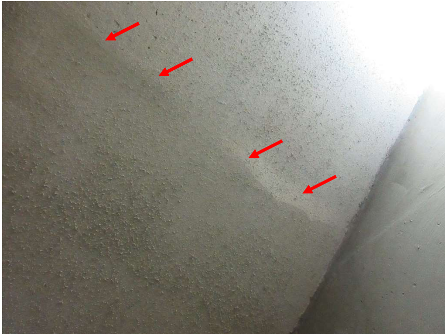
Photo 42 – Distress in finishes on soffit of stair stringer
