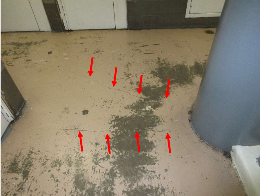
Photo 23 - Cracking in slab top surface at Level 9
