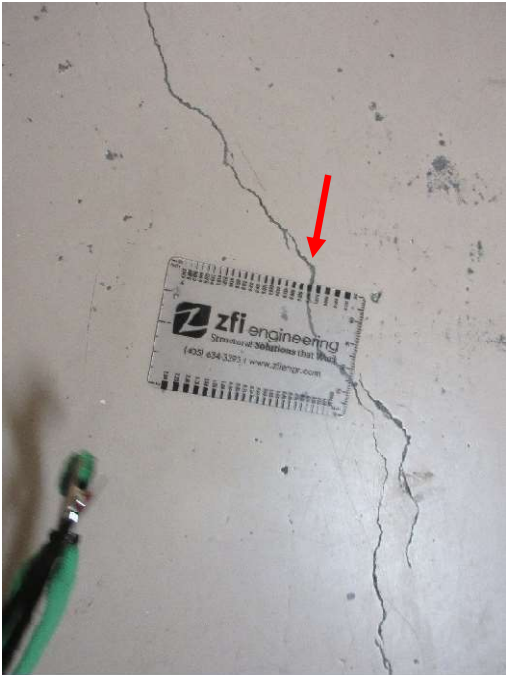
Photo 10 - Approximate width (0.060") of crack in slab top surface at Level 13
