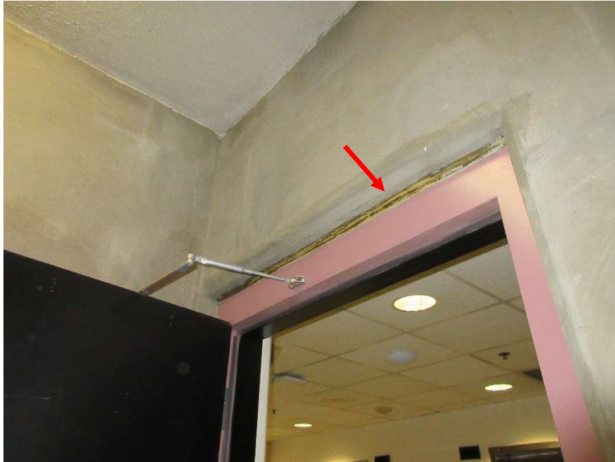
Photo 39 – Distress at door frame of stairwell
