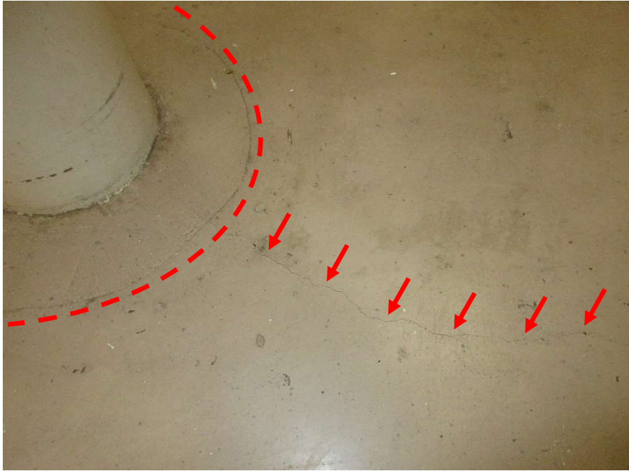
Photo 19 – Circular construction joint & cracks at Level 12
