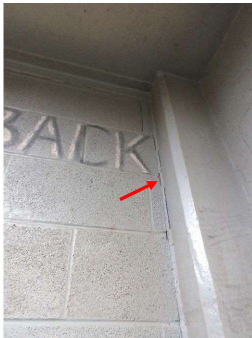
Photo 38 – Cracking in sealant of vertical joint at cell wall
