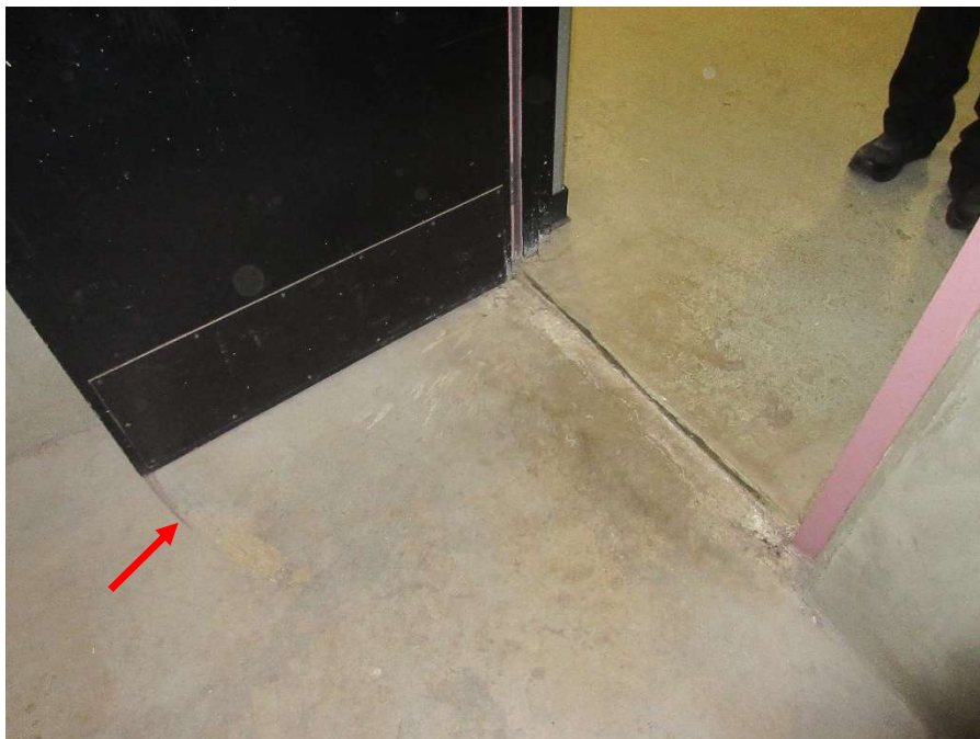
Photo 40 – Abrasion in floor surface from door at stairwell
