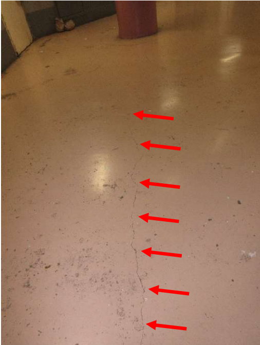
Photo 11 - Cracking in slab top surface at Level 10
