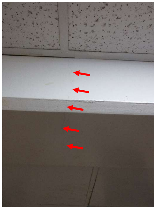
Photo 6 – Hairline crack in rectangular beam at Level 14
