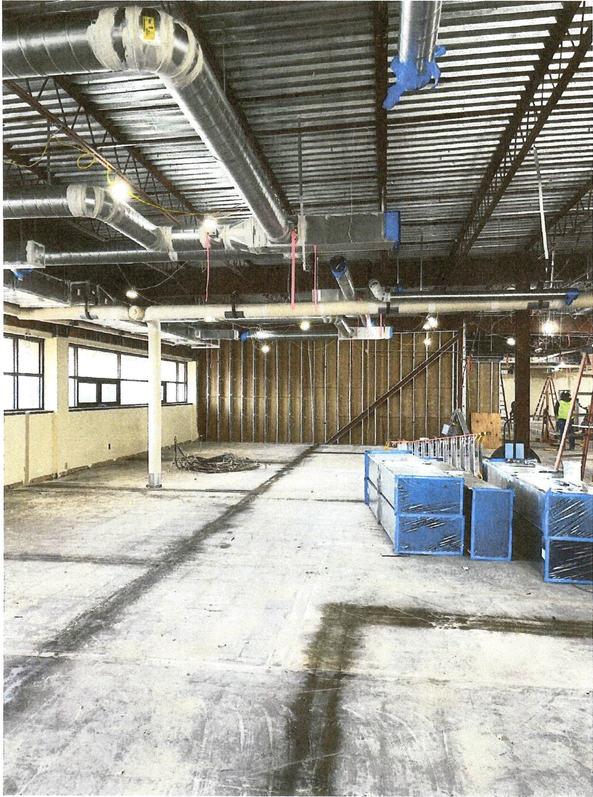
Krowse existing building mechanical
