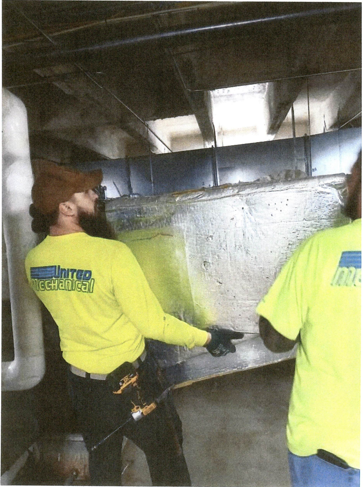
Detention Center 7 th Floor Duct
