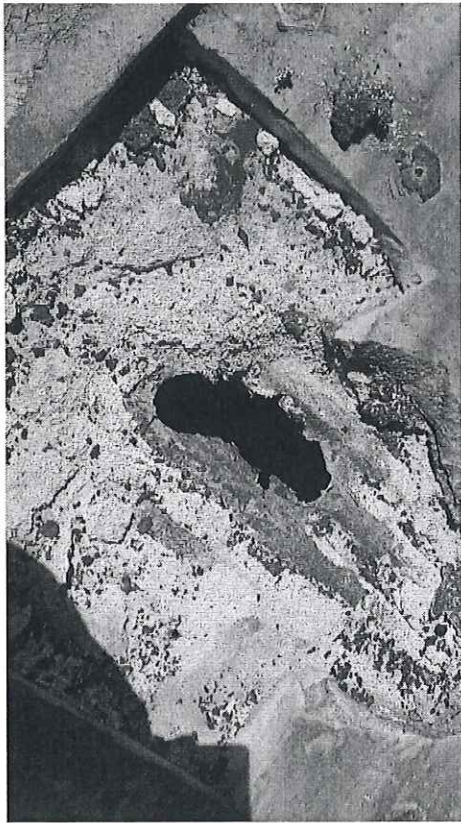
Figure 3: Damaged Roof Deck
